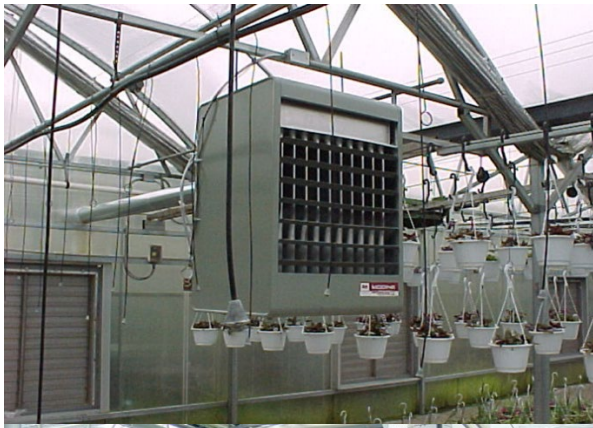
Gas-fired unit heater that blows hot air into the greenhouse production area.
