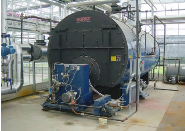
Gas-fired boiler that delivers hot water to the greenhouse production area.
