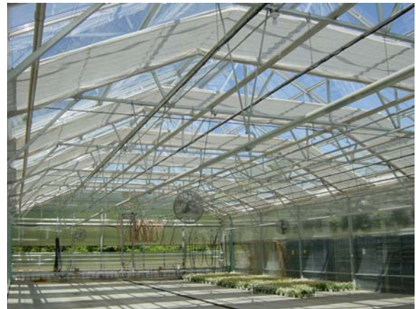
Figure 4. Internal shade system.
