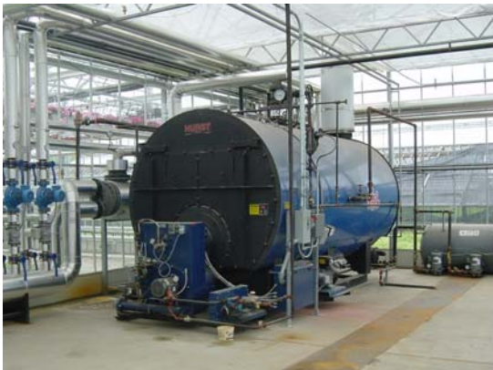
Photo 2. Hot water boiler at Cromwell Growers, Cromwell, CT.
