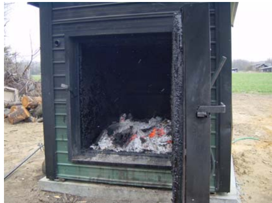
Photo 3. Wood boiler at Weaver's Farm Market, Pittsgrove, NJ.
