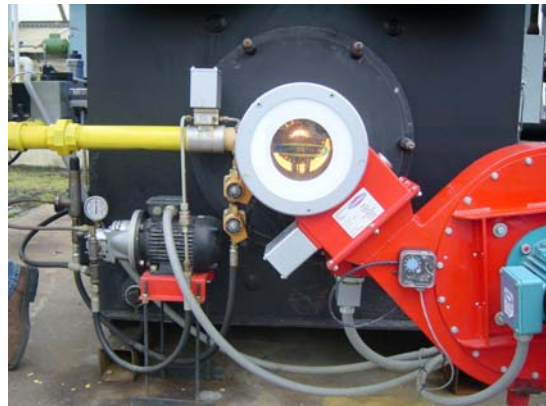
Photo 4. Dual fuel boiler at Kube Pak, Allentown, NJ.
