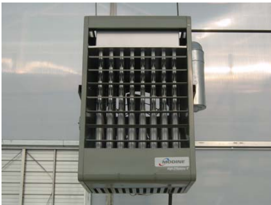
Photo 1. Unit heater at Lucas Greenhouses, Monroeville, NJ.
